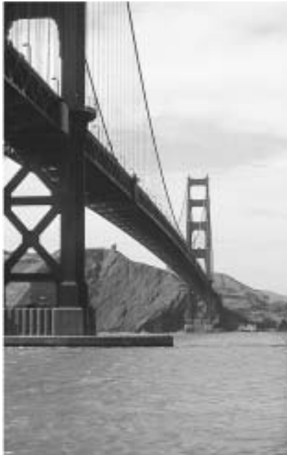
FIGURE 3.6 The Golden Gate Bridge in San Francisco—one example of an exquisite arrangement of balanced forces on the structure.
